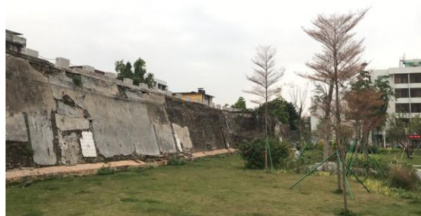
Figure 6. Environmental Status of the City Wall in Nanxi Road Section.
