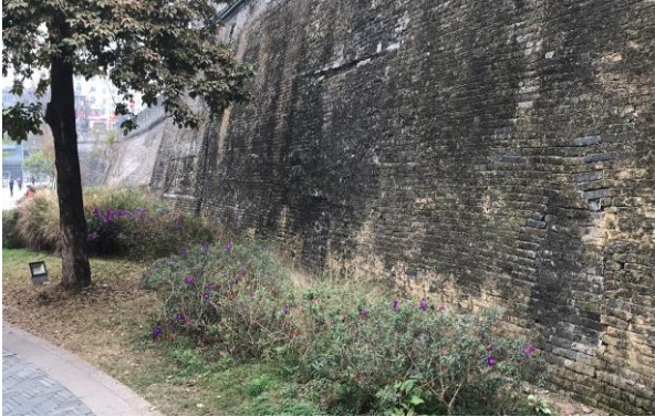
Figure 1. Environmental status of Songcheng Road I.
